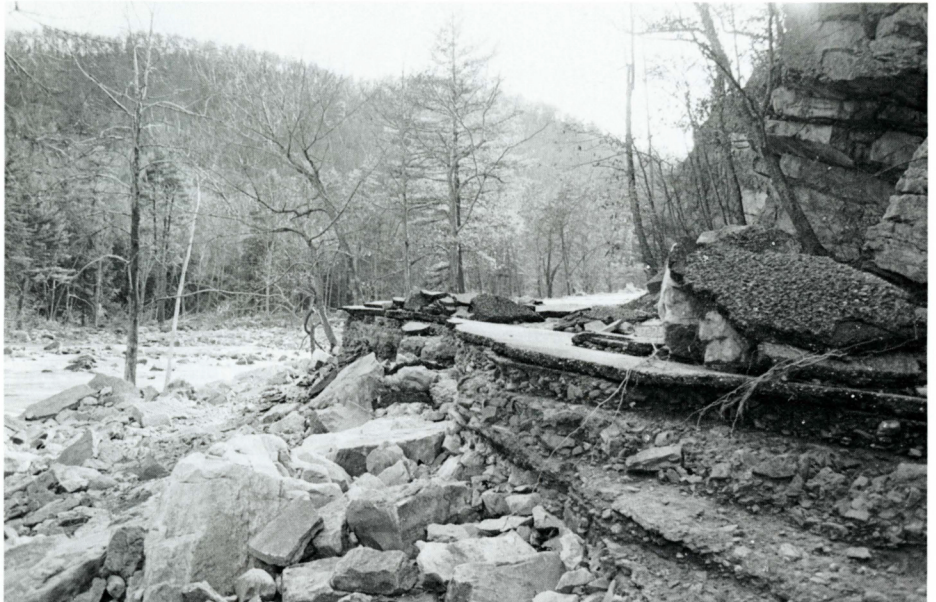
The road through Goshen Pass, a familiar byway for Washington and Lee students, was torn asunder by flood waters of the raging Maury River. Goshen was one of the areas hardest hit by the November flooding.
